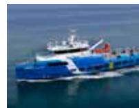
GRANDWELD SHIPYARD - Offshore crew boats: ECOMar 8 STP System
